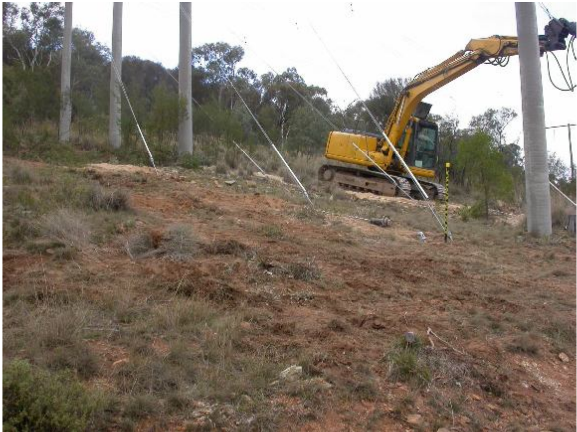
Figure 5 Replacement of power pole stays. Mt Majura nature reserve, June 2009. Implementation and maintenance of utilities highly impact on conservation and recreational values.
